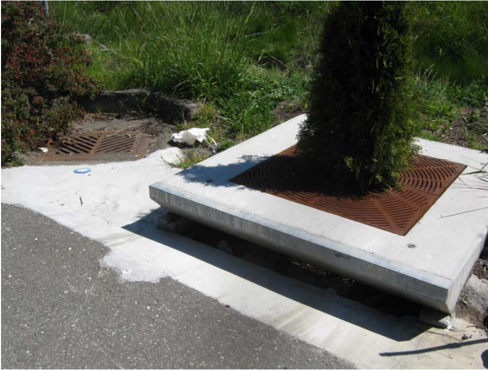
Photo 10. Stormwater control structure for parking lot of Freeland Park.
