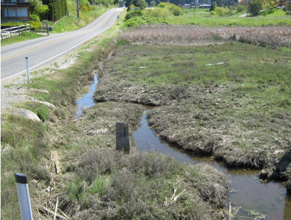
Photo 4. Pocket estuary located south of Shoreview Drive and west of South Woodard Avenue. Looking south from roadway above outlet culvert.
